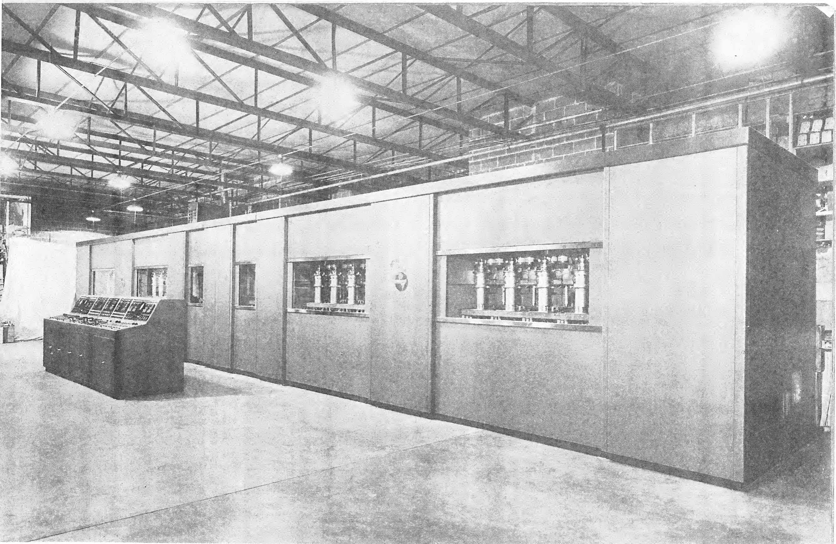
The Main Assembly of the Type 105-C, 1000 kw, Transmitter Including the Control Console
